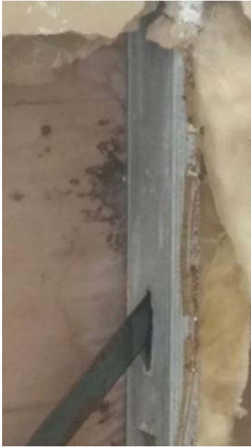
Photo 1: St. John's Lane Room 79 – Mold and Water Staining
