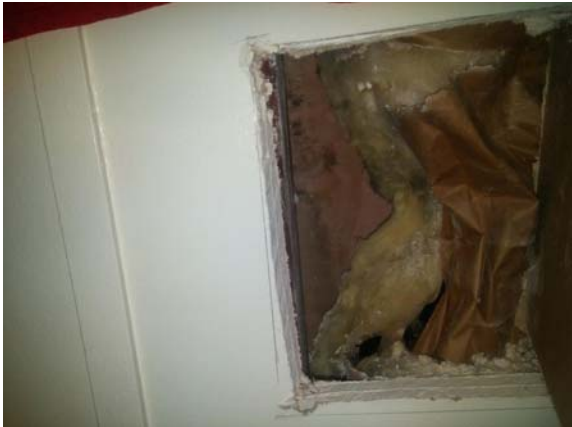
Photo 13: St. John's Lane ES Room 83 Test Cut – Presence of Mold and Water-Impacted Materials
