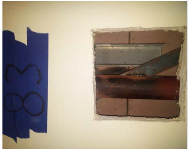
Photo 14: St. John's Lane ES Room 83 – After Cleanup and Encapsulation with Shockwave Sanitizer
