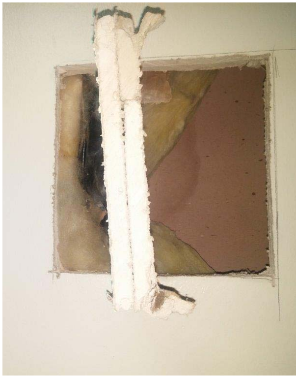
Photo 11: St. John's Lane Room 82 Test Cut on South wall – Presence of Mold and Water-staining
