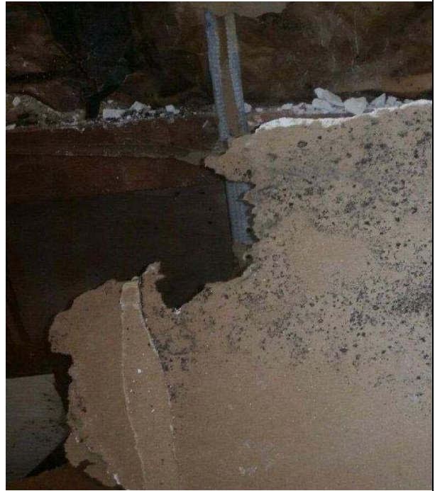
Photo 2: St. John's Lane Room 79 – Mold on the Drywall
