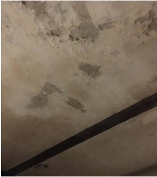
Photo 9: St. John's Lane Library Room 102 Above Doorway – Mold on the Roof Deck Drywall
