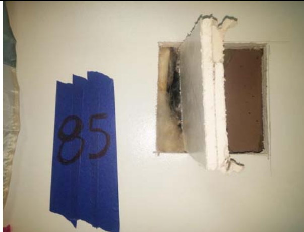
Photo 17: St. John's Lane Room 85 Test Cut – Presence of Mold and Water-staining
