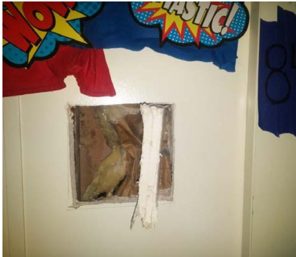
Photo 15: St. John's Lane Room 84 Test Cut – Presence of Mold and Water-staining
