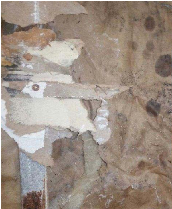
Photo 3: St. John's Lane Room 79 – Mold on the Batting Insulation and Drywall
