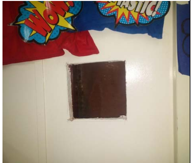
Photo 16: : St. John's Lane Room 84 Test Cut– After Cleanup and Encapsulation with Shockwave Sanitizer
