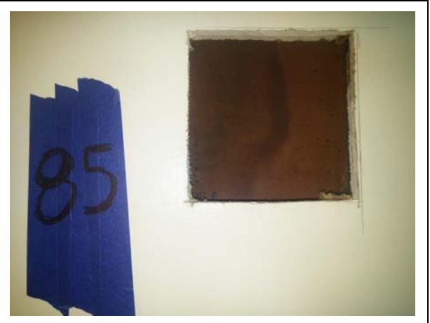
Photo 18: : St. John's Lane Room 85 Test Cut– After Cleanup and Encapsulation with Shockwave Sanitizer
